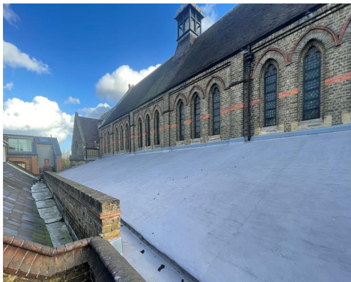
North aisle and middle Church Hall concrete roof, newly solar paint protected
